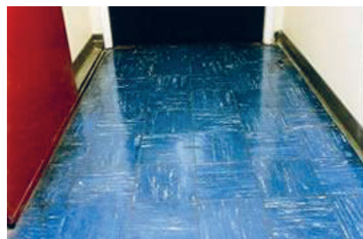
Asbestos containing floor tiles in a corridor
