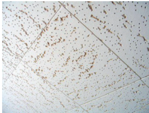
Asbestos containing ceiling tiles
