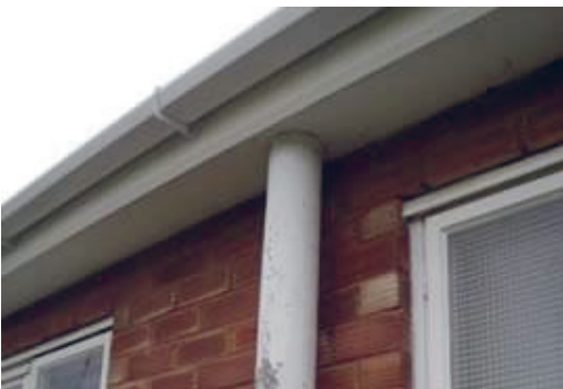
Asbestos cement drainage pipe (downpipe)
