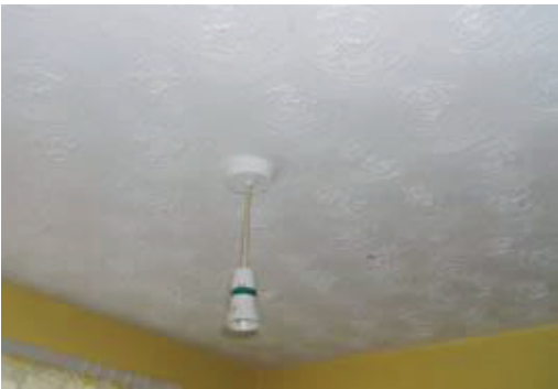
Asbestos textured coating
